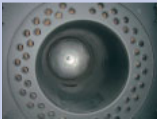
Internal view of combustion chamber
